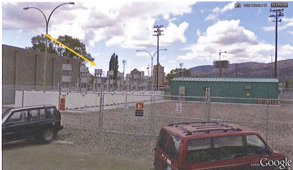
Figure 3 – Static VAR Compensator located at the Recreation Substation in downtown Kelowna
